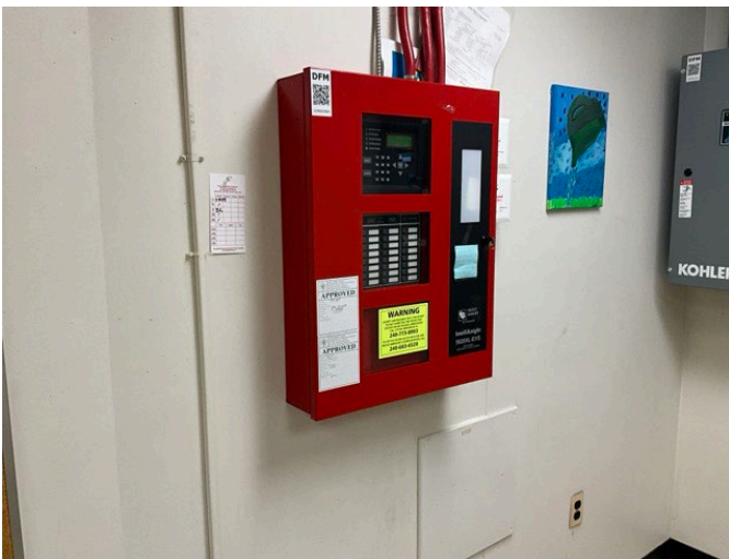
21 - FIRE ALARM SYSTEM
