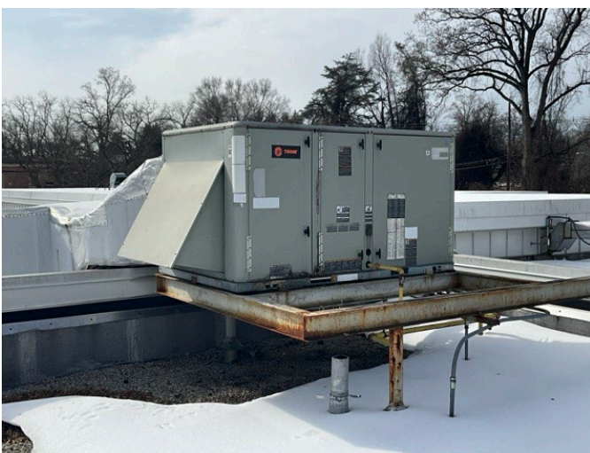
23 - ROOFTOP PACKAGED UNIT
