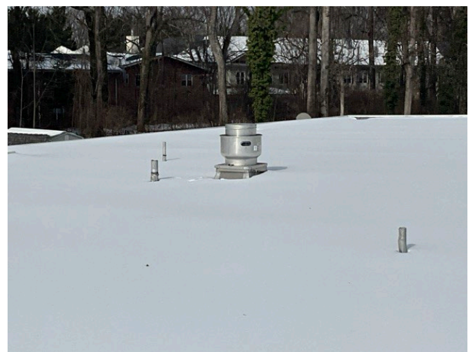
24 - TYPICAL EXHAUST FAN
