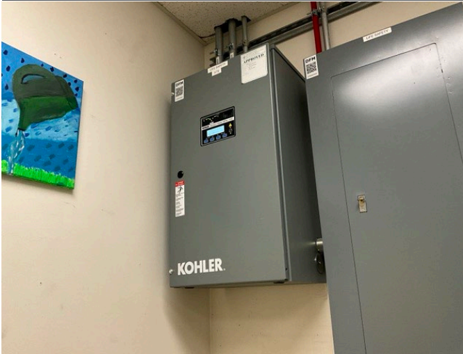
19 - AUTOMATIC TRANSFER SWITCH
