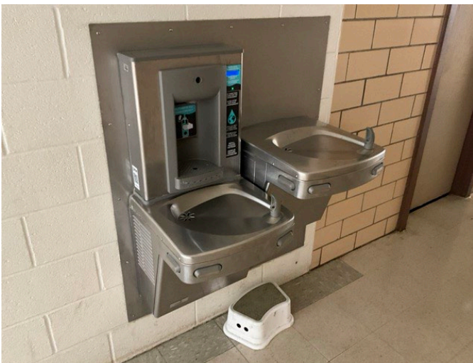
15 - TYPICAL WATER FOUNTAIN
